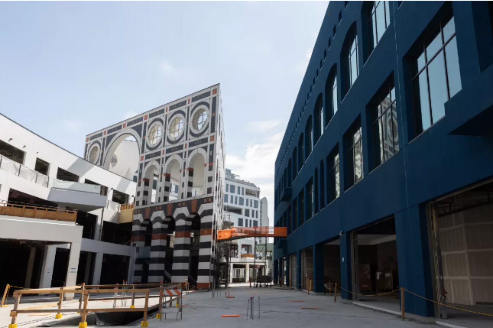
Construction progress at the Campus at Horton in downtown San Diego in late July 27. (Kristian Carreon/For The San Diego Union-Tribune)
